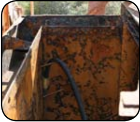
Before: Silo interior surface covered in rust & corrosion
